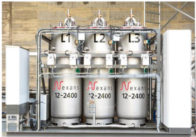
Figure 3 Fault current limiter delivered on site in Essen
