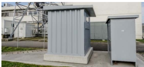
Figure 4 Resistor R_{CC} (left), Selection circuit and circuit breakers (right)
